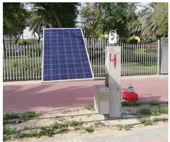
ATS with Terramove Control Box powered by solar panel
